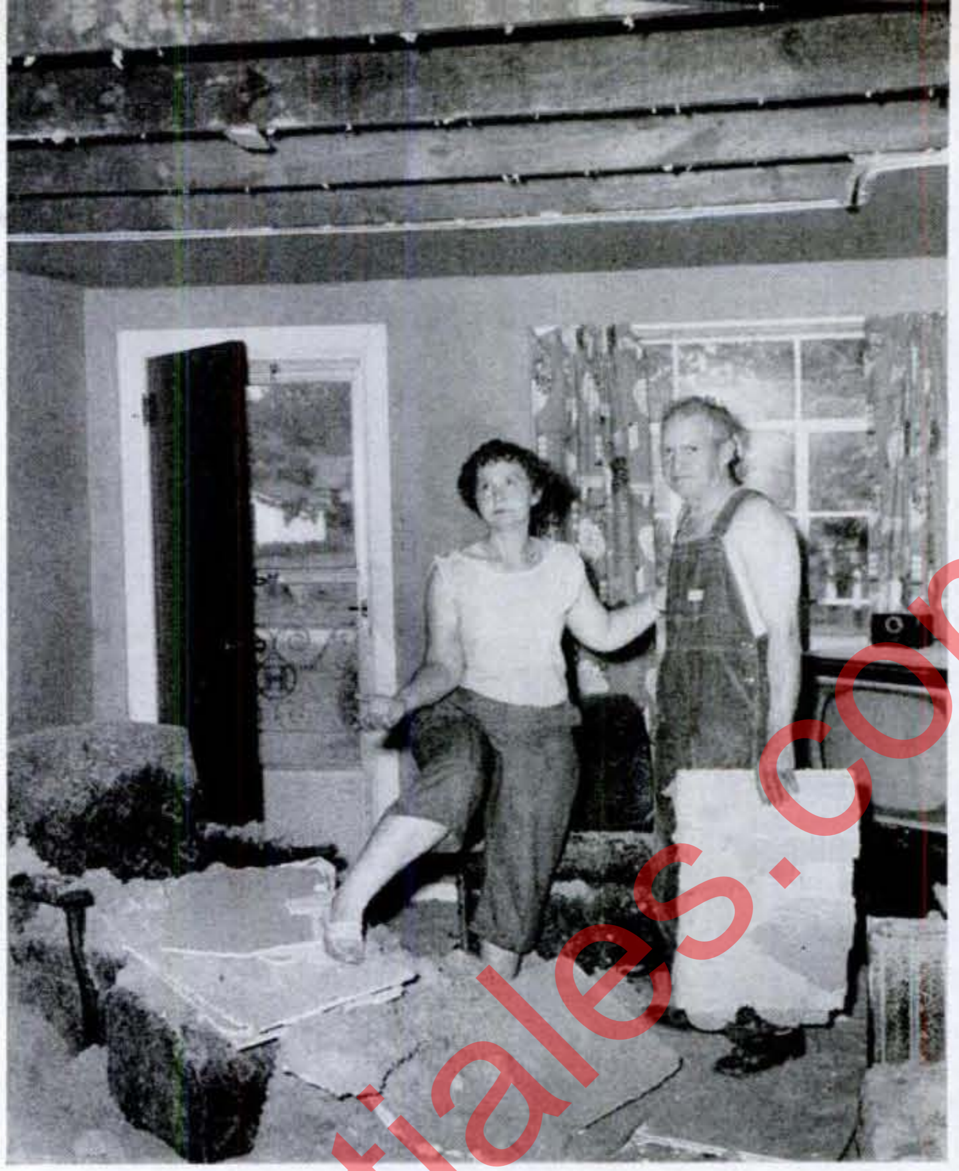
COLLAPSED CEILING in Terre Haute home of Mr. and Mrs. Louis Howerton was result, they claim, of sonic shock wave aimed at ground by descending jet. →
